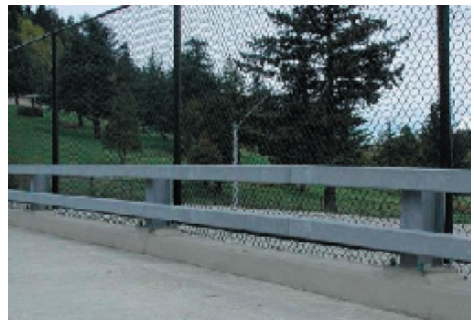
Oregon 2-tube side rail curb mount will be utilized on bridges along the Byway to maintain the open look. A brown color will be utilized (Photo courtesy of FHWA)
