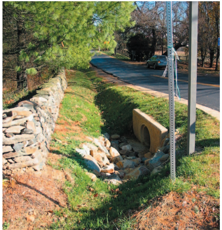
Along Route 50, in Upperville, Virginia, natural field stone was used in lieu of rip-rap and all concrete used for drainage structures incorporated an exposed aggregate finish in order to minimize the contrast with the adjoining stone wall (reconstructed with the same stone as on-site).
